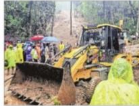
Rescue operations in Kottayam after a landslide on Saturday. PTI
