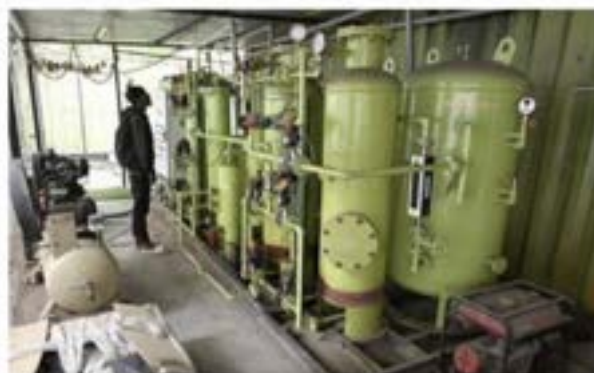
A biogas plant at the Waste-to-Energy unit in Kottamangala in Bengaluru. J. ALLEN GONZALEZ
