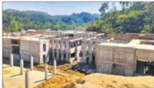
The Assam government constructed the battalion without prior forest clearance and prior environmental clearance. MOEFCC REPORT
